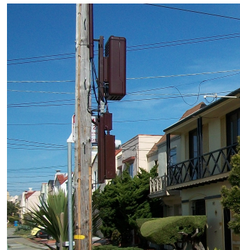
Figure 1: Microcell Cabinet in San Diego
